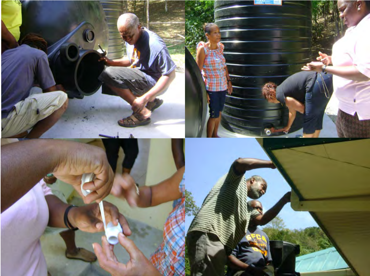
Community teamwork during installation of rainwater harvesting system in Caura Valley. Equipping the community members with new skills provides sources of additional income while building resilience and promoting climate adaptation measures among the wider local community. Photo credit: CANARI
